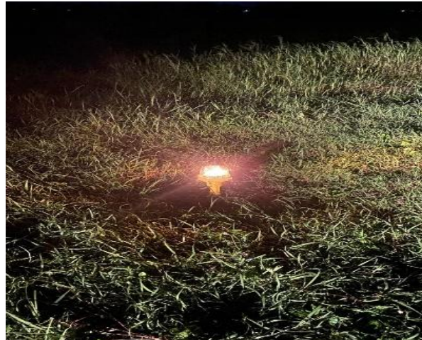
Figure 4. Halogen lights on Runway 14 of Kertajati International Airport, West Java
